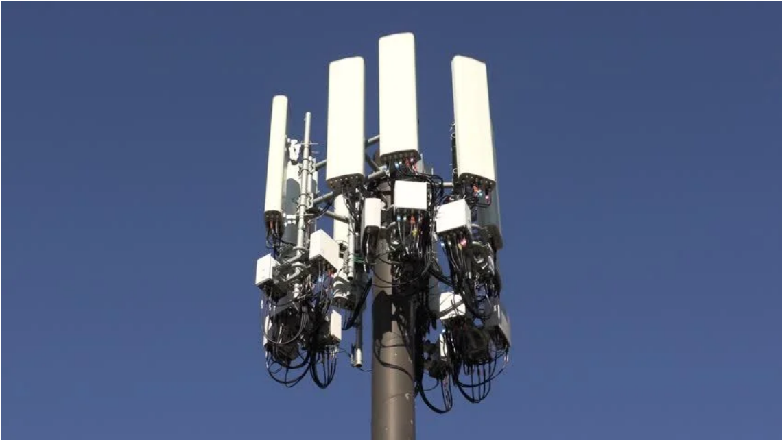
Figure 3.6: 5G antenna tower
