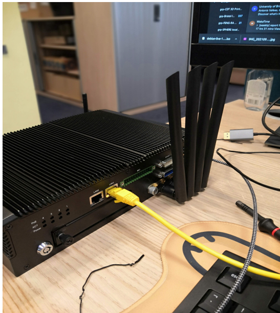
(a) Indoors router
